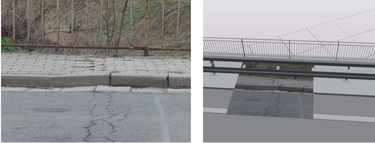
Figure 5.11: Representation of some cracks at the pavement as a texture depicted on a plane.
