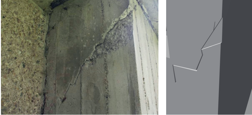
Figure 5.12: Representation of a spalling at the abutment.
