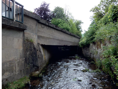
Figure 5.6: Photo of the bridge for case study. The photo has been provided by the "Thüringer Landesamt für Bau und Verkehr".
